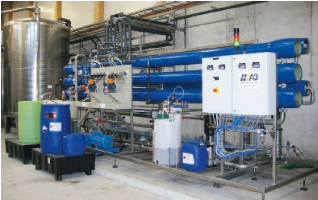
Figure 2: Permeate-stepped reverse osmosis plant
